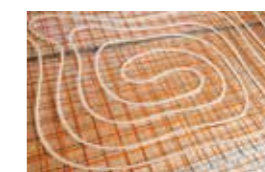
Floor heating loop
